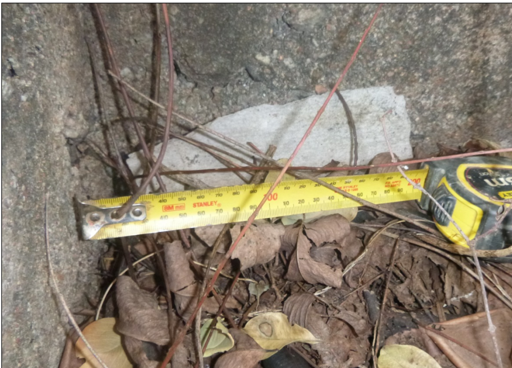
Figure 6: Possible bonded ACM, in sound condition, on concrete footing in northern part of site
