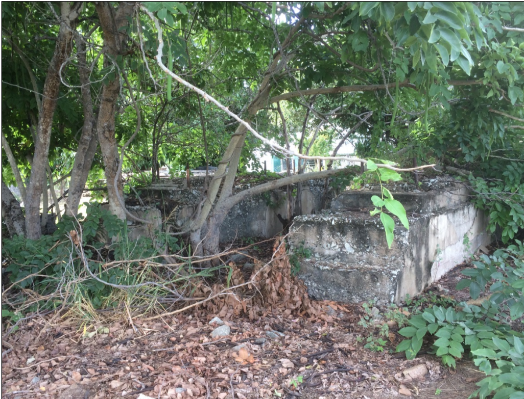
Figure 5: Concrete footings, located under the trees. Photo taken from centre of site, looking north
